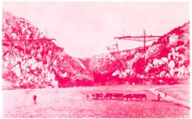
Blaauwkrantz bridge on the Grahamstown to Port Alfred railway line under construction.
